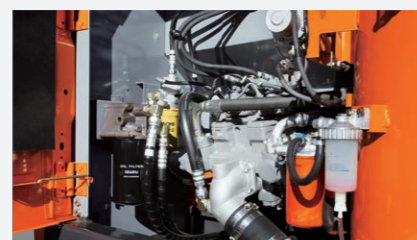
Grouped remote filters and inspection points
