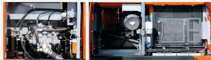
Grouped remote filters and inspection points Utility space and radiators
